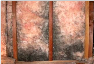
Signs of an Air Barrier issue. Dirty insulation or drywall in the cavity.
