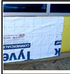
Typical Issue during masonry tie installation.—which needs to be corrected.
