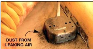
Signs of an Air Barrier issue. Dirty drywall or wood in the cavity.
